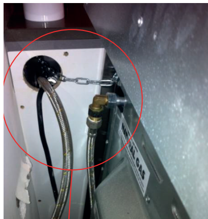
Hole in cabinet is too large, allowing the upright cooker to tilt forward
